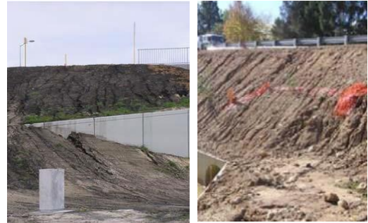
Soil surface erosion following earthworks
