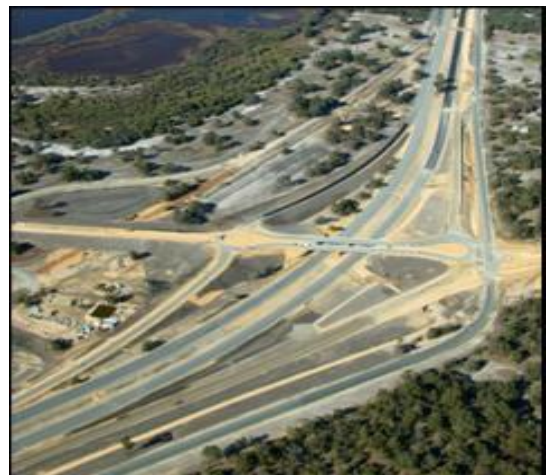
View of project area with locations designated for the stockpiling of site materials
