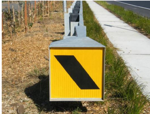
Photograph of SKT – SP installation
