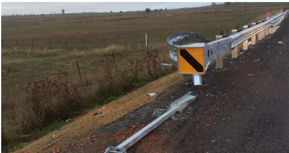
Photograph showing W-Beam extruded onto verge side
