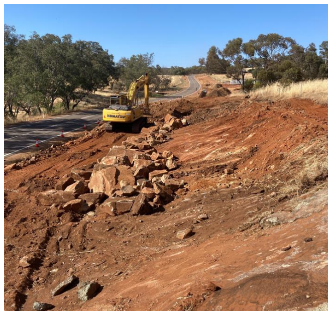
Vegetation and rock removal works adjacent to the eastbound carriageway of Toodyay Road
