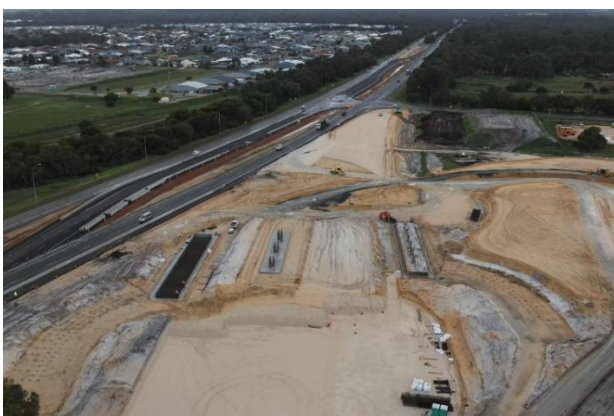
Construction site for the Paris Road and Clifton Road interchange next to Forrest Highway with CMC columns being constructed
