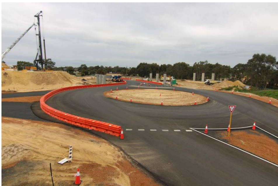
Recently completed concrete columns at the 'mega-bridge' construction site near Golding Crescent
