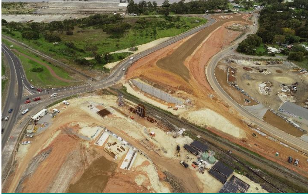
Temporary road layouts and interchange construction at Hanrahan Road / Frenchman Bay Road
