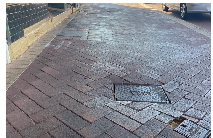
Some level differences in pavement around services create trip hazards
