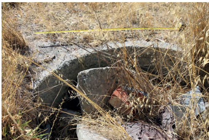
IMG_0014 .....400143 mE 6483918 mN Septic tank with terracotta pipe
