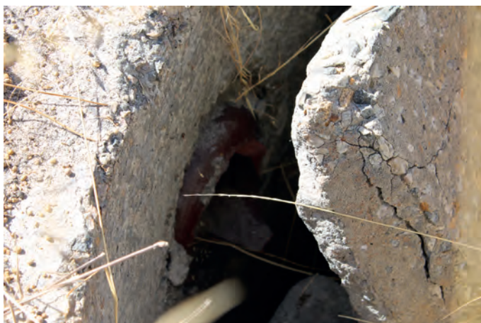
IMG_0016 .....400143 mE 6483918 mN Septic tank with terracotta pipe
