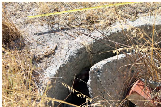
IMG_0015 .....400143 mE 6483918 mN Septic tank with terracotta pipe
