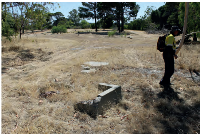
IMG_0052 ..... mE mN View with Darren Cooper of finished but broken concrete 'wall'
