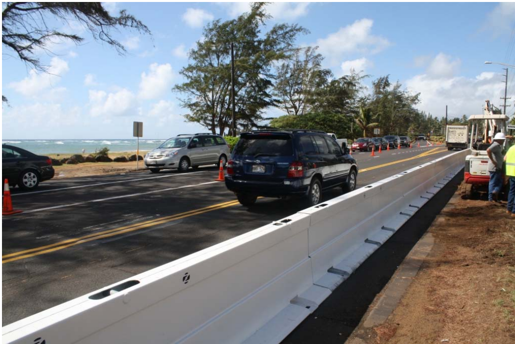
Photograph of Zoneguard installation
