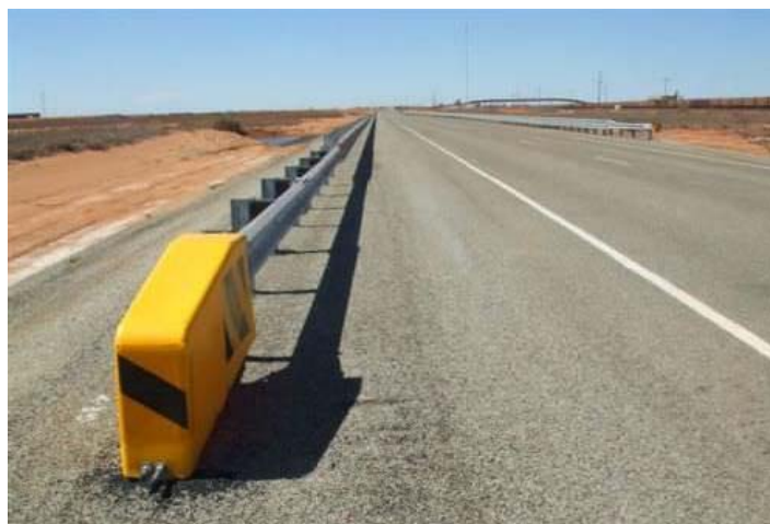
Note sticker is not to Main Roads WA requirements
