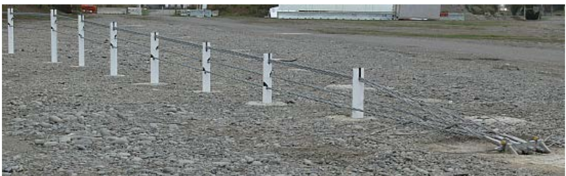
Photograph of Sentryline III end terminal installation.
