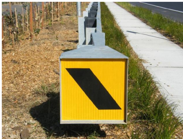
Photograph of SKT – SP installation
