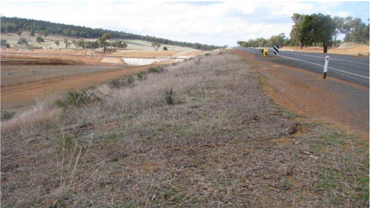
Figure 1. Roadside Batters Prior to Rehabilitation in 2012.
