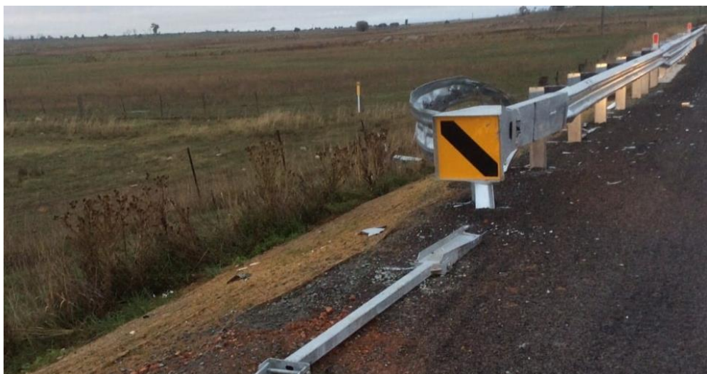
Photograph showing W-Beam extruded onto verge side
