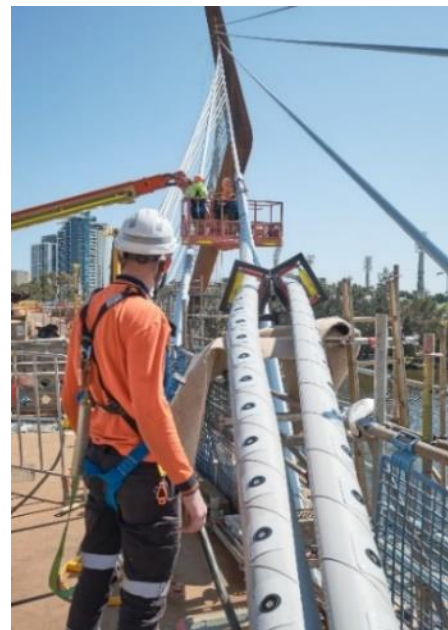
Figure 3: An outer duct with LED lights being installed on the cables at Point Fraser
