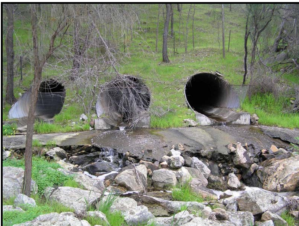
Photo 4 - UNDERMINING OF APRON ON RHS
