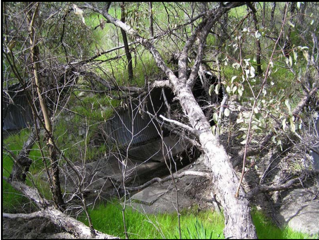
Photo 3 - WATERWAY PARTIALLY BLOCKED BY TREE AT INLET (LHS)
