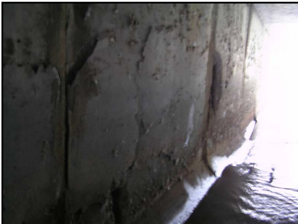
Photo 6 - TYPICAL DELAMINATION AND SPALLING OF CULVERT UNITS
