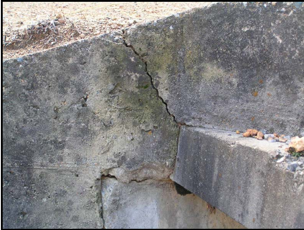
Photo 5 - CRACK BETWEEN RHS WING WALL 1 AND RHS HEADWALL
