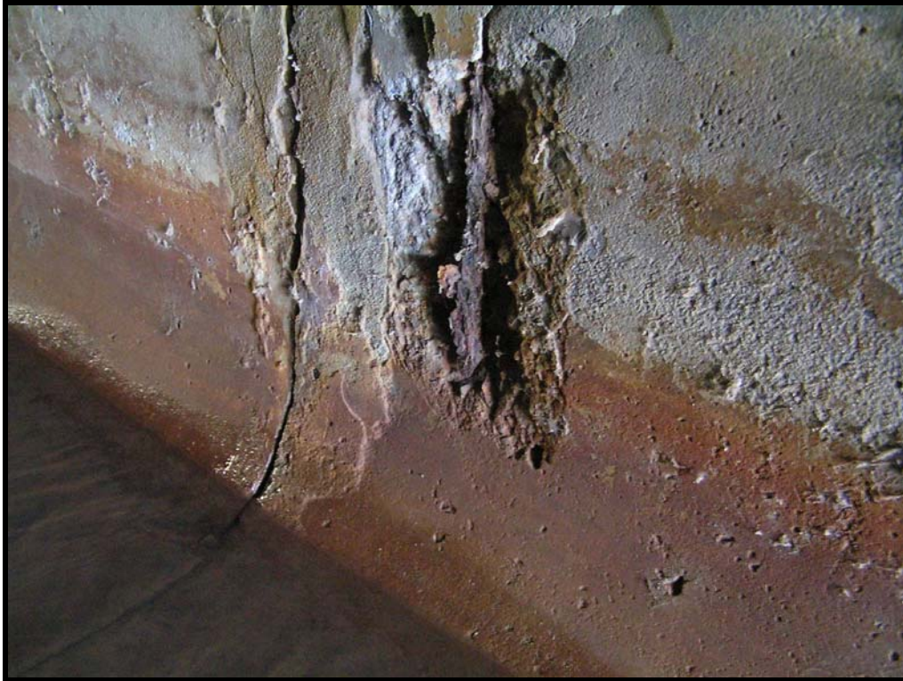
Photo 7 - TYPICAL CORROSION OF REINFORCEMENT IN CULVERT UNITS
