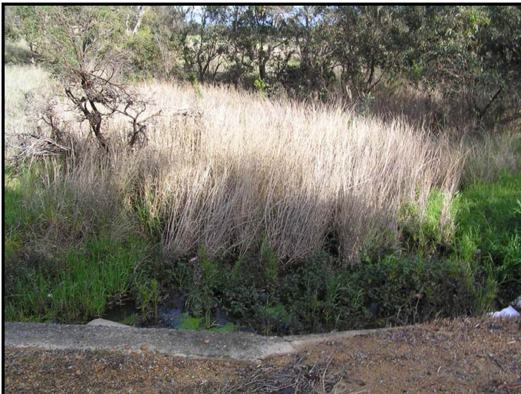
Photo 4 - VEGETATION RESTRICTING FLOW ON RHS
