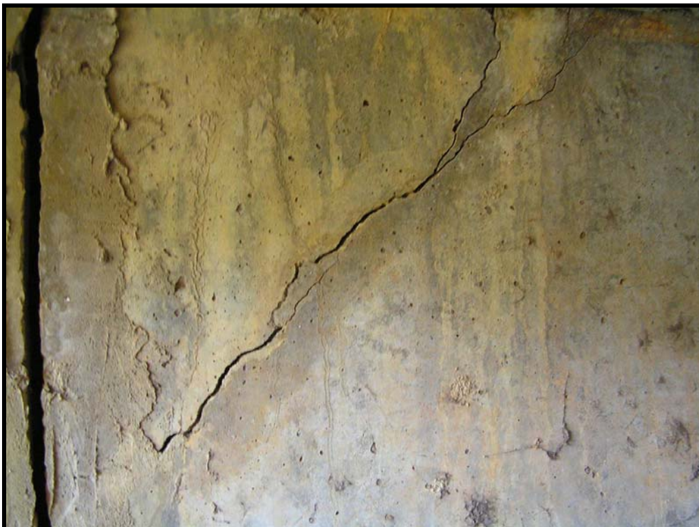
Photo 8 - 4 mm CRACK BARREL 2, UNIT 2, A2 SIDE
