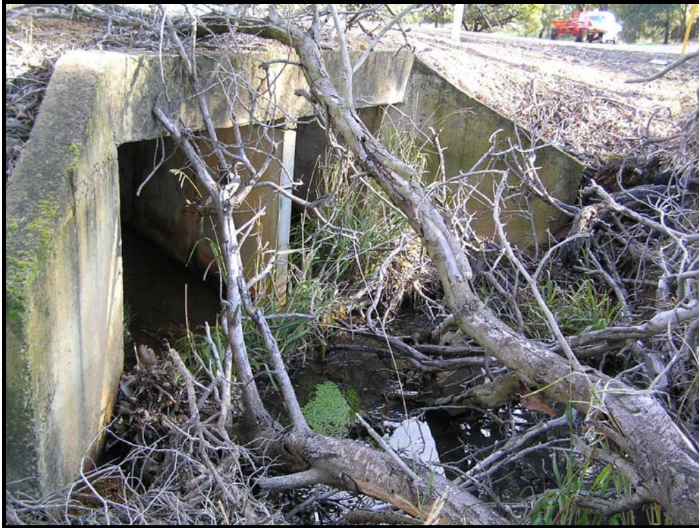
Photo 3 - BUILD-UP OF DEBRIS AT INLET (LHS)
