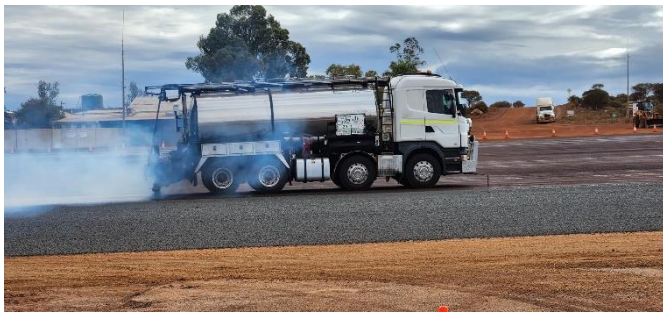
The Mid West-Gascoyne Region complete sealing work opposite the Paynes Find Roadhouse on Great Northern Highway.
