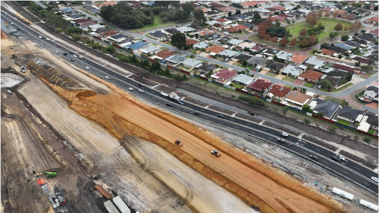
Figure 10 The orange-coloured material represents the Brajkovich fill material at Altone Road
