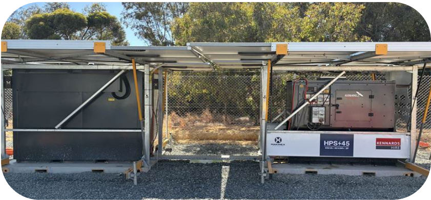
Figure 6. Hybrid off-grid power system at Mundijong site office
