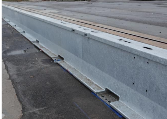
Photograph of Installation
