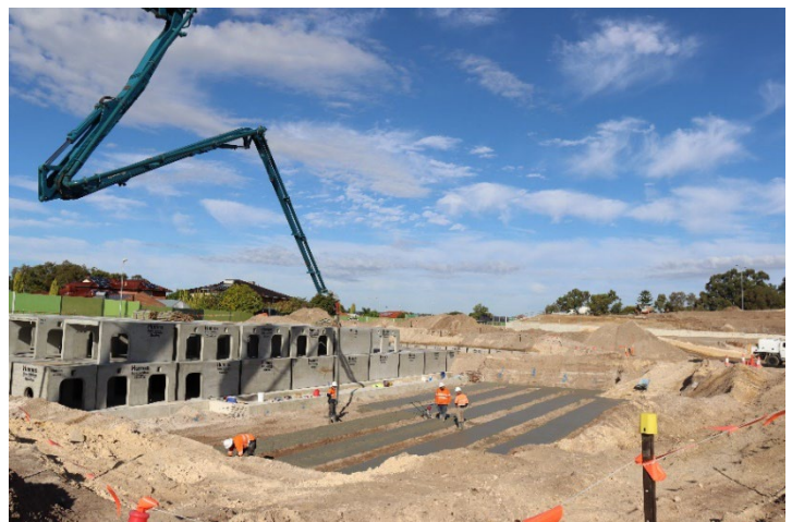
Noranda Station carpark storm traps.
