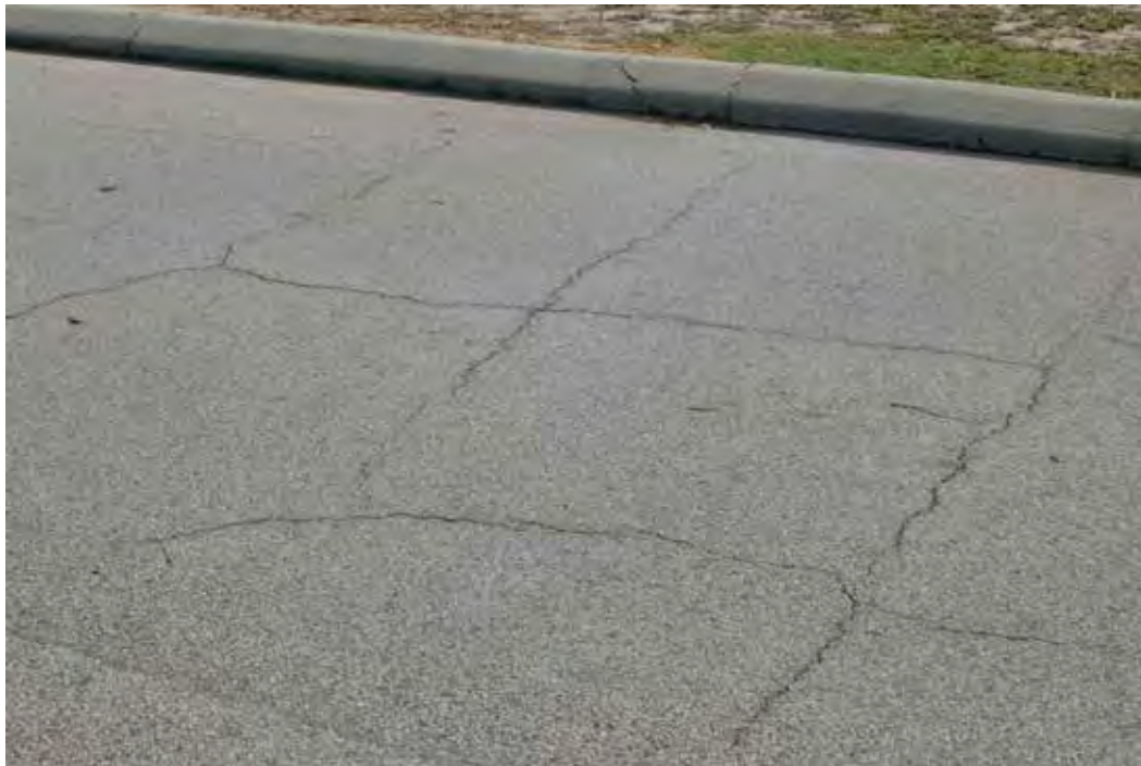
Figure 15: Block cracking on local streets.
