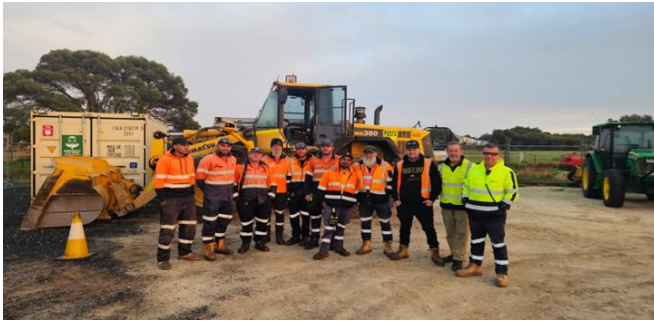
Yonga Civil and Main Roads team members on site at Forrest Hwy Intersection & Access to Glen Iris project, marking a strong start to Yonga Civil's work in the South West region.
