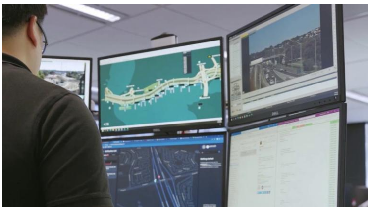
Figure 9-1: The RNOC control room
