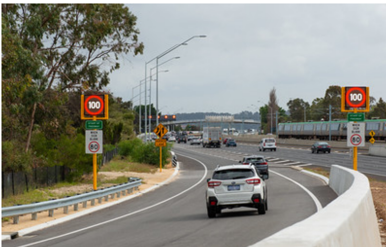
Figure 6-2 Example of side mounted VSL sign
