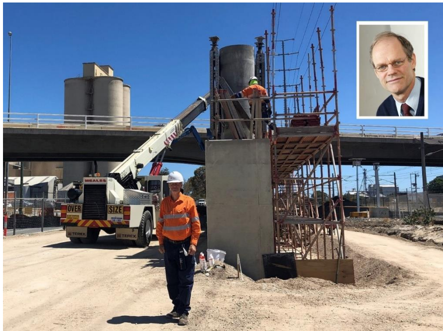
Tale of two bridges: Engineer Graeme Dundas in front of the duplicate bridge under construction, with the existing bridge in the background.
