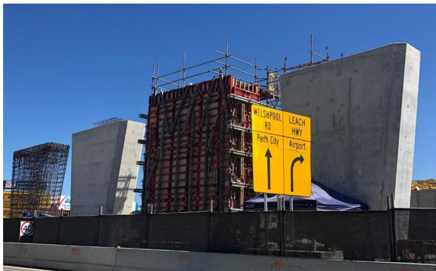
Under construction: Piers for the new Leach Highway bridge over Welshpool Road.
