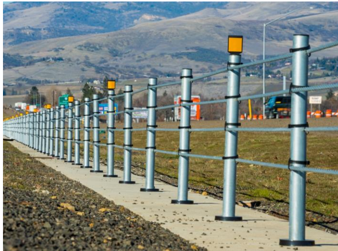
Photograph of MASH TL3 BRIFEN wire rope safety barrier installation (concrete strip footing shown).
