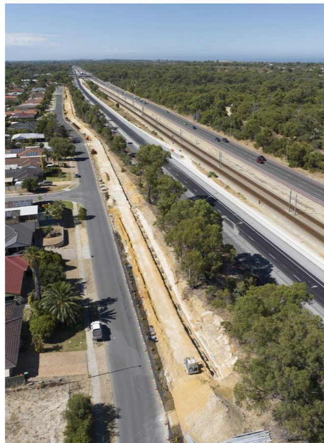
Figure 1 Aerial view of works along Camarino Drive showing the Principal Shared Path and Freeway works.
