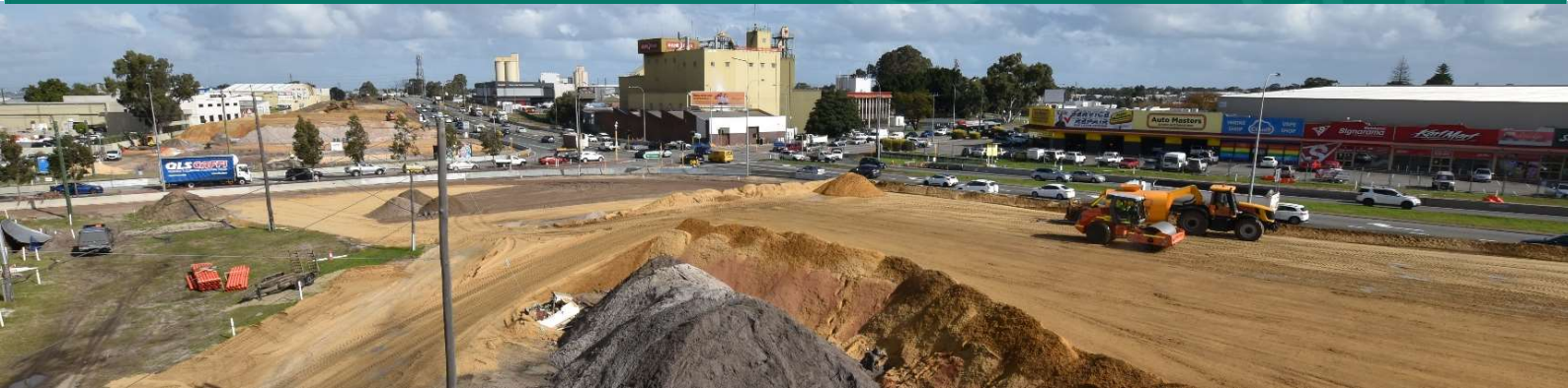
A time-lapse image of works at the north east corner at the Leach Highway and Welshpool Road intersection (6 July 2021)
