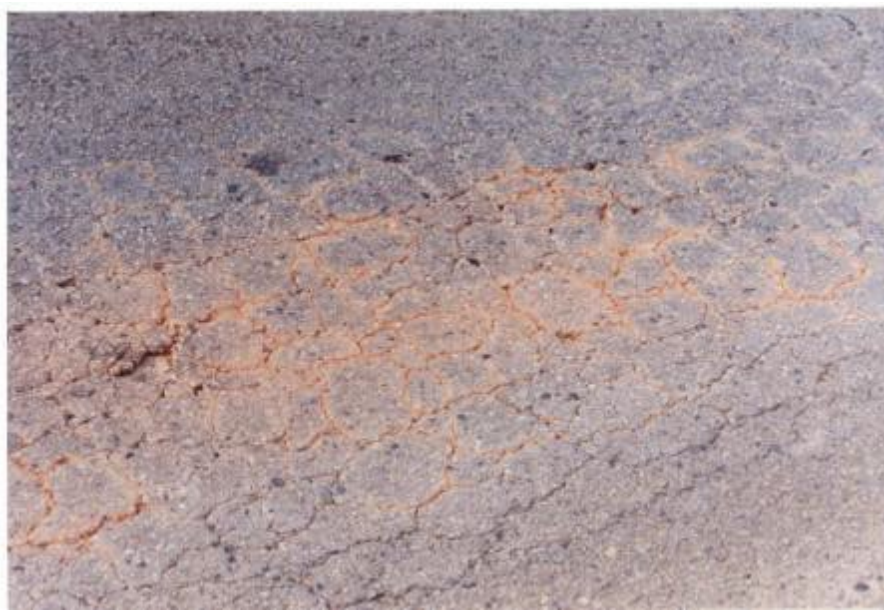
HIGH SEVERITY structural cracking with pumping
