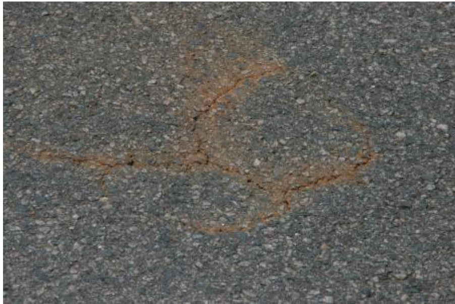
HIGH SEVERITY Environmental unstable cracks
