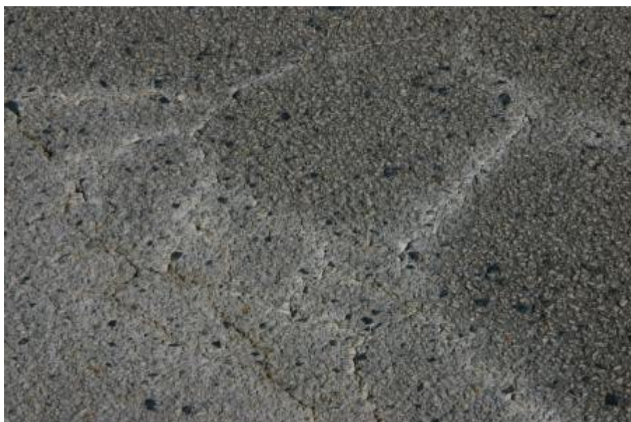
HIGH SEVERITY Environmental unstable cracks
