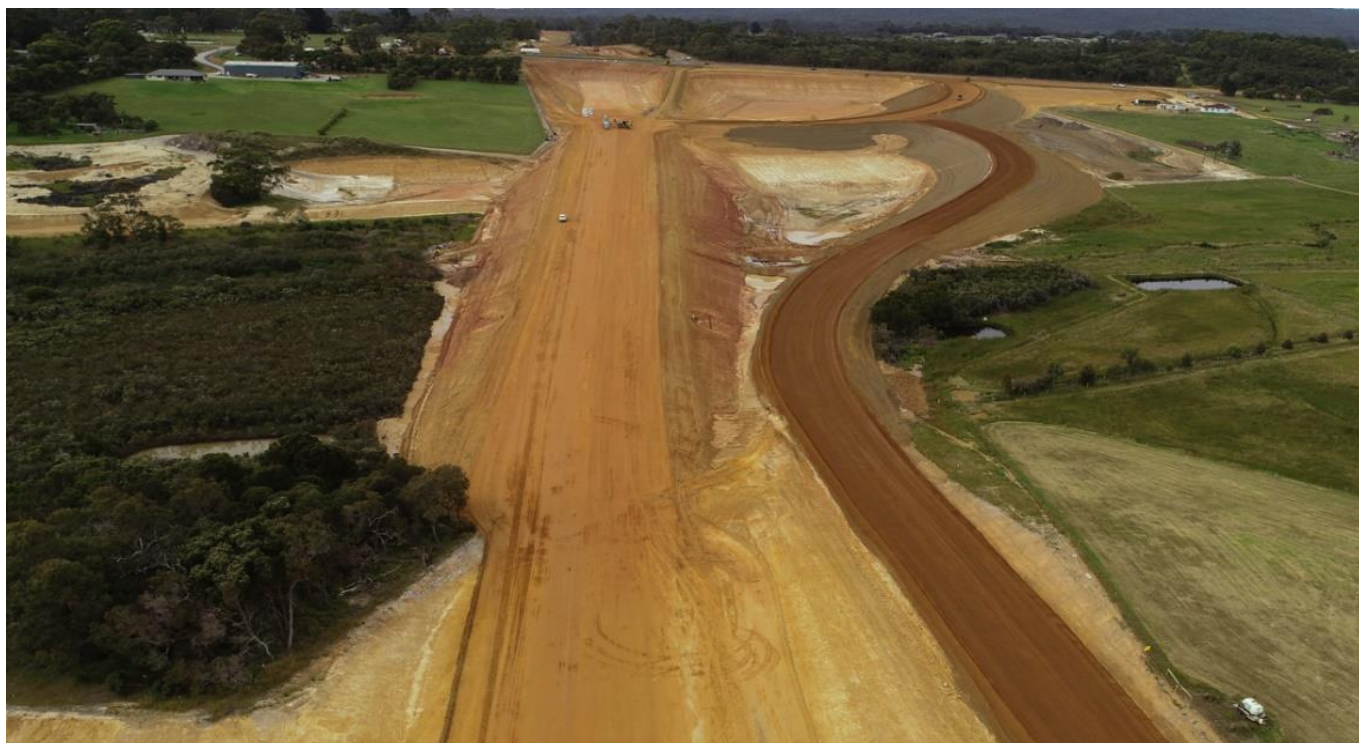
Earthworks at the Albany Ring Road, Link Road and South Coast Highway interchange (looking south towards South Coast Highway)
