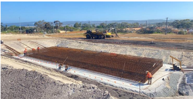
Abutment footing preparation at the Hanrahan Road / Frenchman Bay Road bridge site
