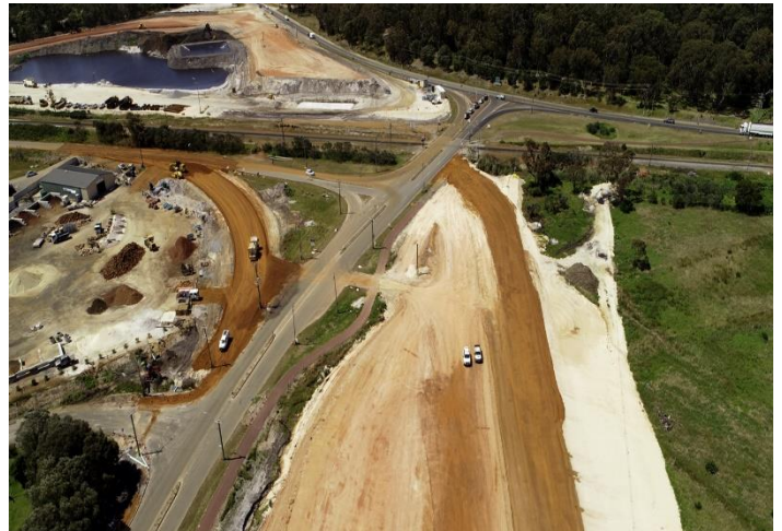
Earthworks at the Hanrahan Road / Frenchman Bay Road interchange site (looking north towards Hanrahan Road)
