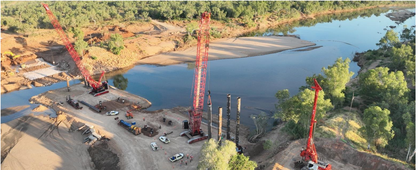
Above: The bridge team driving piles into the riverbed to provide support for the bridge.
