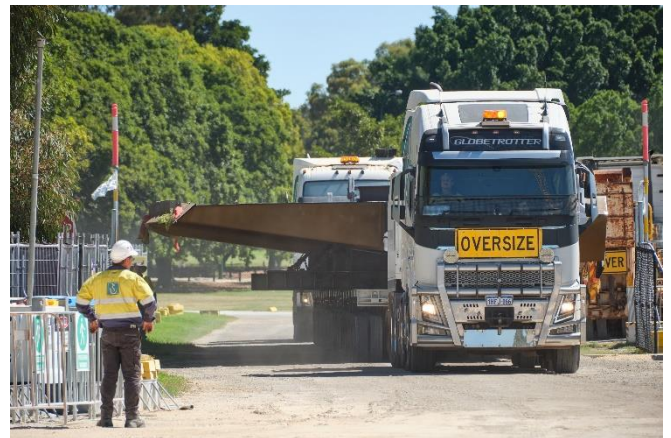
Figure 5 The first of the fabricated bridge deck segments’ being delivered to site.
