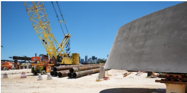
Figure 10 Installation of the segments, pylons and pile caps is complex and will involve a range of crane lifts (dual and single). Images shows one crane, fabricated piles and a pile cap shell on site at McCallum Park.
