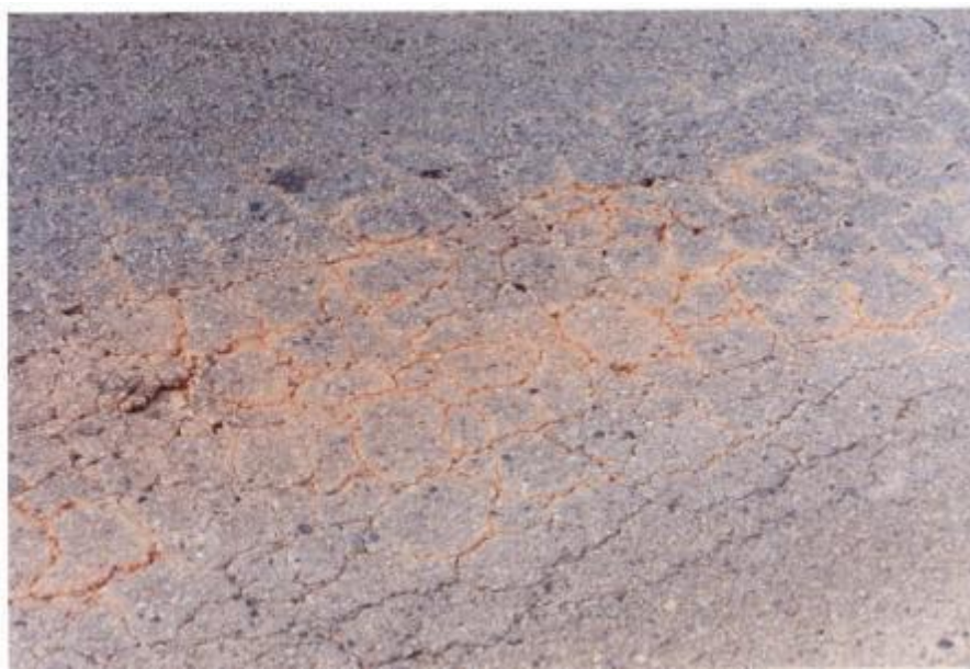
HIGH SEVERITY structural cracking with pumping
