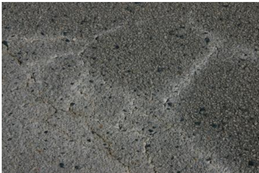
HIGH SEVERITY Environmental unstable cracks
