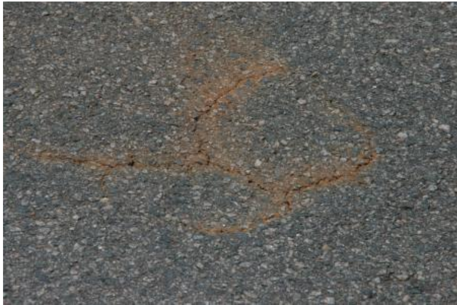
HIGH SEVERITY Environmental unstable cracks
