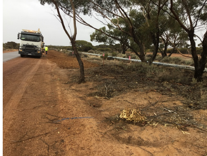
Photograph 2: Demarcation and topsoil stripping in location of Dampiera glabrescens prior to clearing
