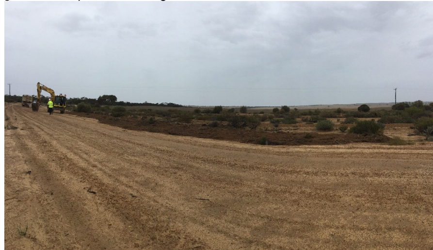
Photograph 4: Respread of topsoil to 5 cm thickness in cleared area of revegetation offset site
