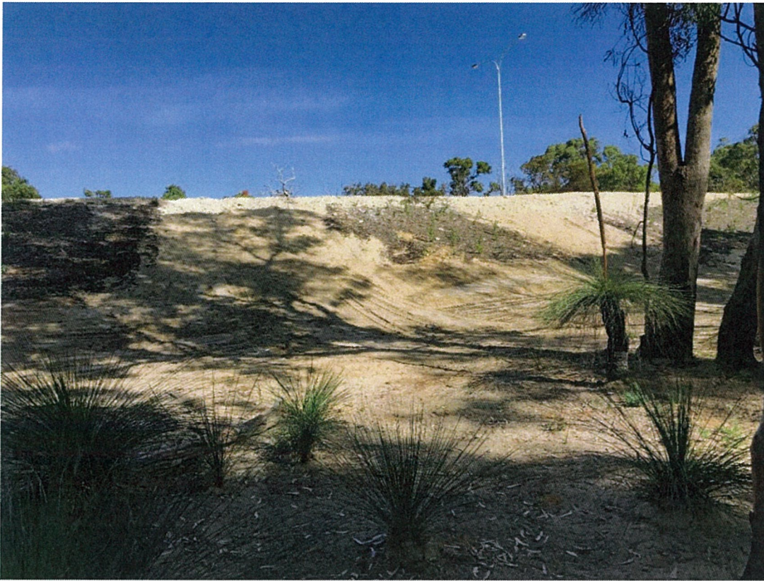
Photo A.1 Location of erosion and sediment control incident, occurred 31/1/2017
