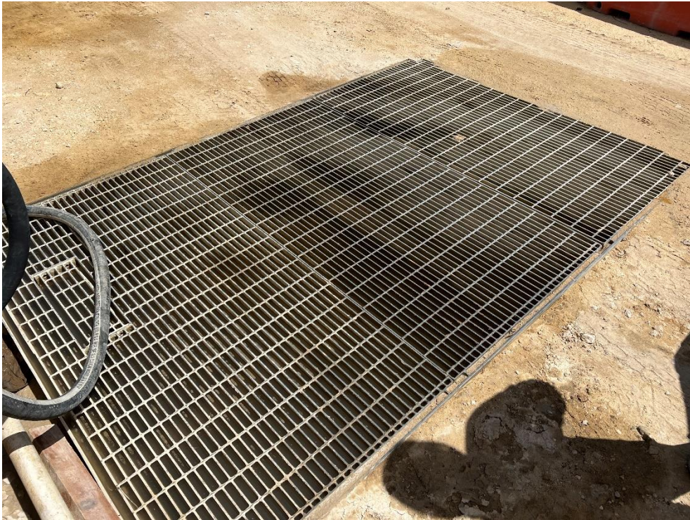
Observation No. 1 – bund at refuelling station full of rainwater
