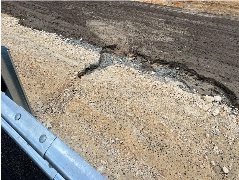
Scour observed from recent rain events
