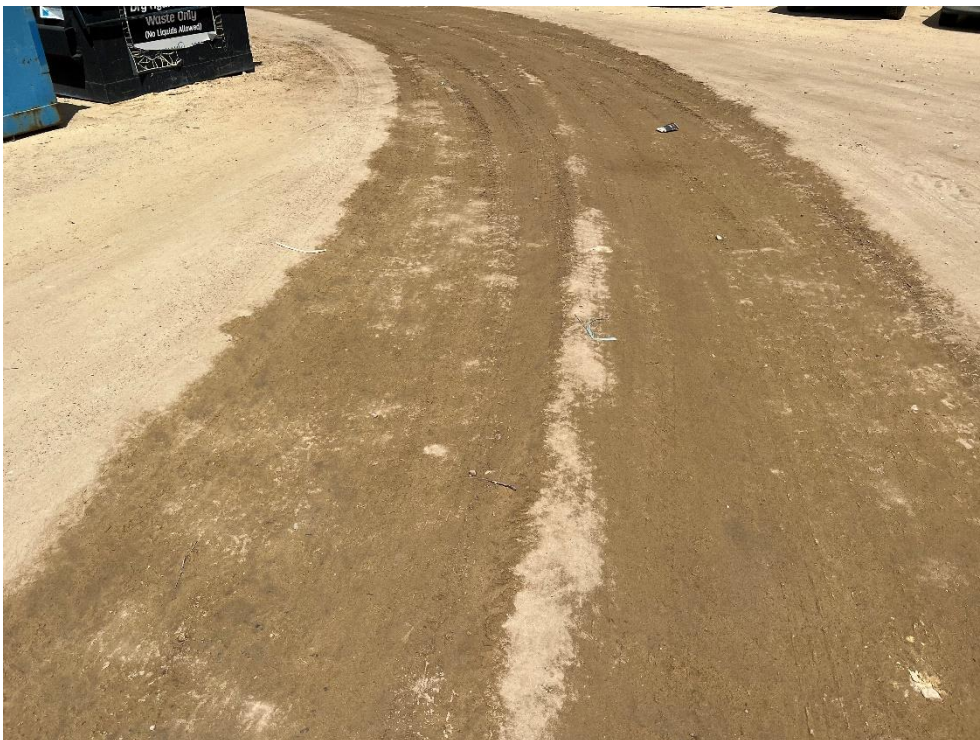
Main access route through Lukin Dr compound damped down with a dribble bar
